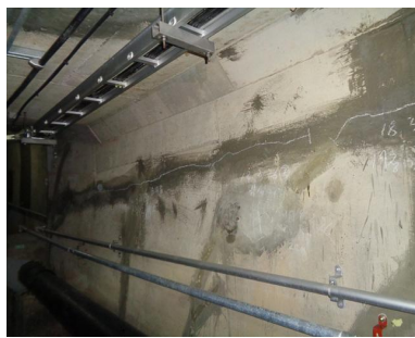
Sta.760~780m Type ② 균열 0.1/5.8
