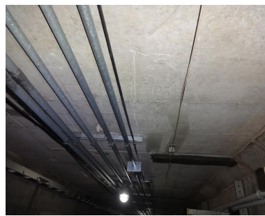
Sta.860~880m Type ① 균열 0.1/0.7
